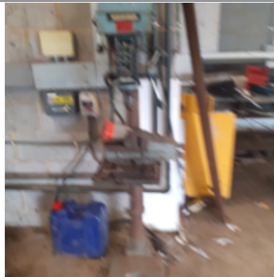
1x Floor Mounted Pedestal Drill
